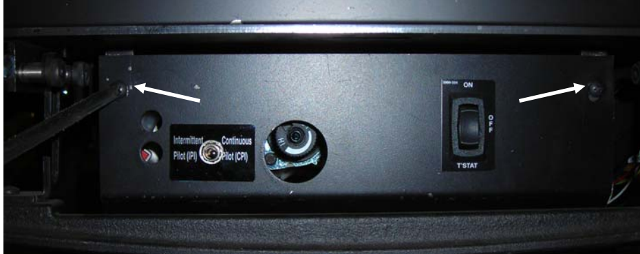
Photo 15 – Modesty Panel Removal
