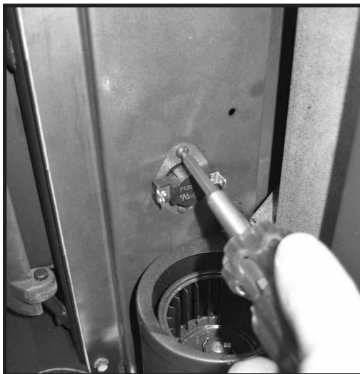
Figure 20: Removing thermal switch.
